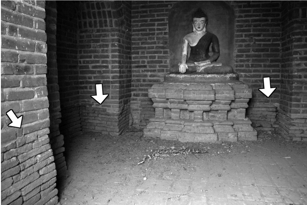
Plate 2 Temple 1130C. Interior rebuilt in 1998 above original walls (arrowed). The brick pedestal with a reproduction of a Bagan-style brick and plaster Buddha image have been rebuilt over the core of the original pedestal. (Photo 2008.)
