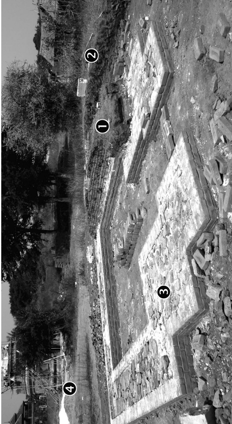
Plate 3 Mound 2779, with excavated foundation (1) and new brick footings (3), set to be rebuilt as a temple. A separate brick line (2) may be remnants of an enclosure wall. The heap of lime (4) used for mortar for a nearby reconstruction was visible in satellite imagery. (Photo 2008.)
